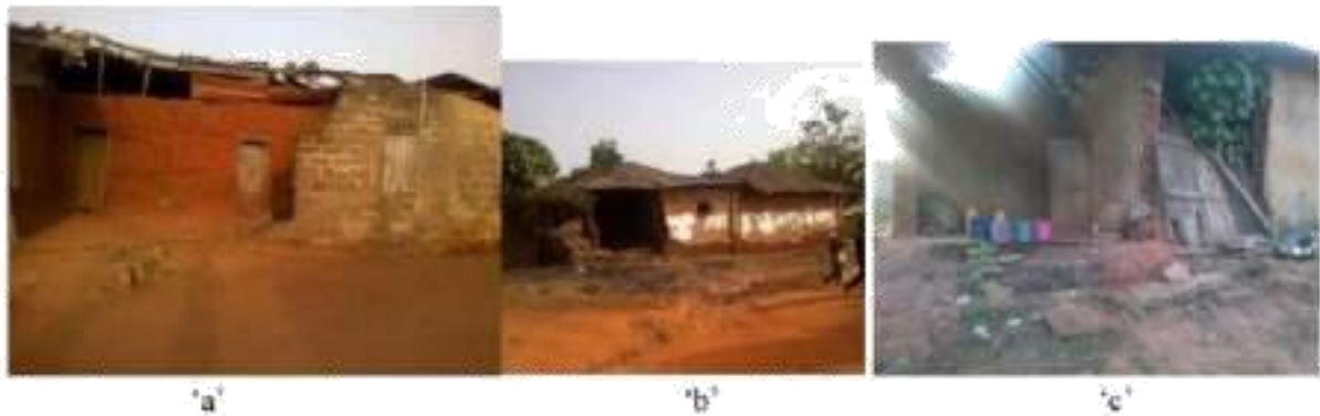
Plate 2: Collapsing Structures that are still dwelling homes (including 'c' with internal weeds).
